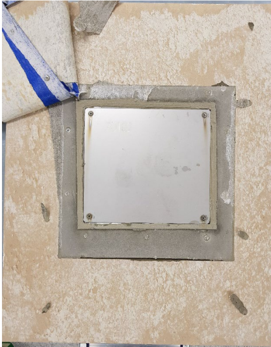
Image 5 – Webertec folie has been removed for inspection of leakage
