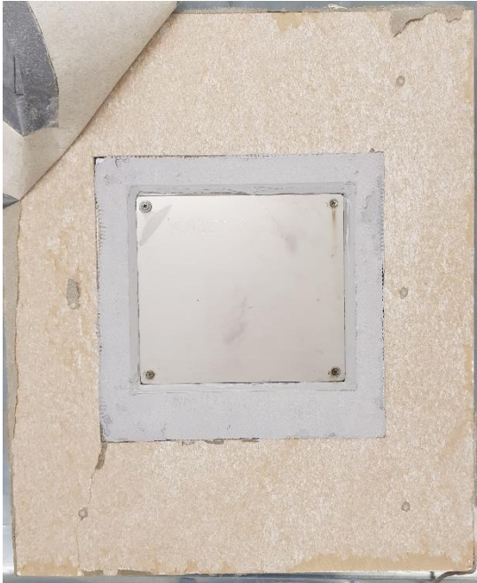
Image 5 – Mira foil Vapourmat 4500 removed for inspection of leakage
