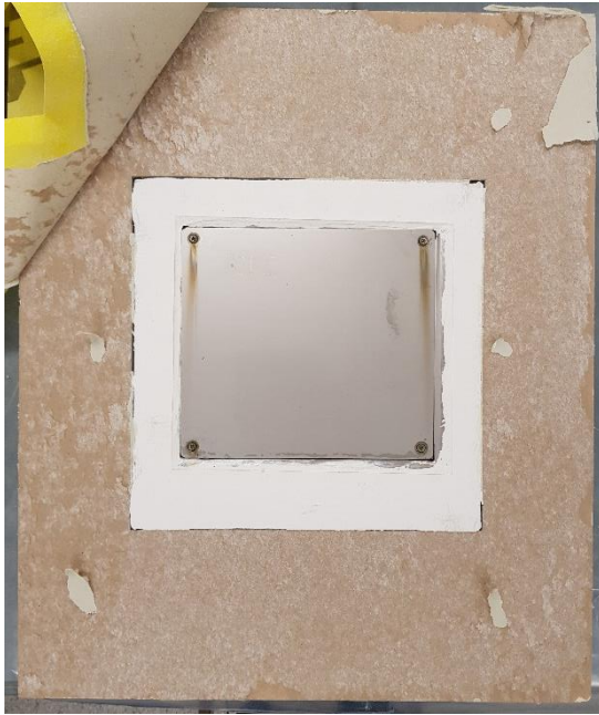
Image 5 – LIP Foil removed for inspection of leakage
